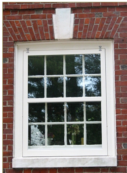
Installed storm window
